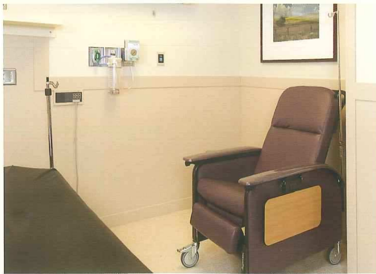
OUTPATIENT SURGERY ROOM CLADDING Chip-resistant Corian® is durable enough to stand up to hard knocks from gurneys, chairs and medical equipment.
